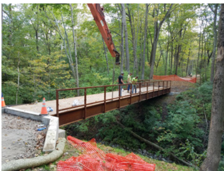
A bridge under construction along a new segment of the Camp Chase Trail in Battelle Darby Creek Metro Park.
