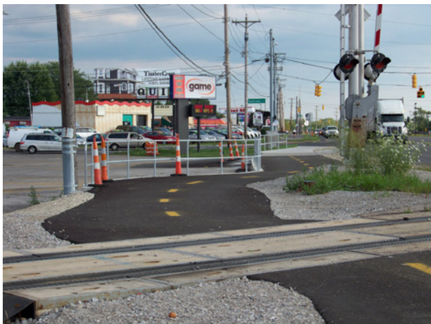
A new section along Georgesville Road in Franklin county was completed in 2019, eliminating a segment of roadway on Industrial Mile.
